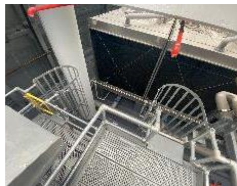
12. Interior, Level 51, Plant Room, Cooling Towers, Upper Level – Guardrail and ladder cage height less than the 1 m prescribed within AS 1657.
