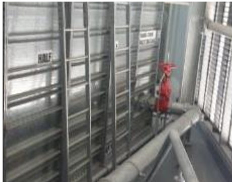
1. Interior, Level 51, Plant Room, Combined Hydrant and Sprinkler Tanks – The front clearance of the rung ladder was obstructed.
