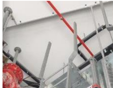
2. Interior, Level 51, Plant Room, Combined Hydrant and Sprinkler Tanks – Restricted headroom at the landing platform / top of tank.
