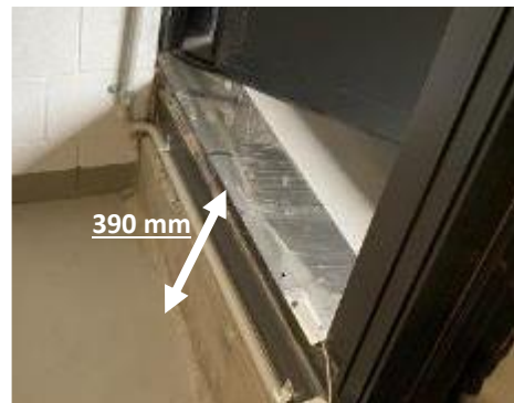
4. Exterior, Podium 3, Plant Room, Balcony – The thresholds/steps at the base of the door frames were measured to extend 390 mm above the ground, presenting trip hazards.
