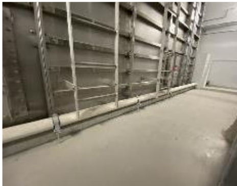
15. Interior, Level 26, Plant Room, Potable Water Tank – PVC pipe obstructing the required 200 mm clearance from the back edge of the rungs of the rung ladder.
