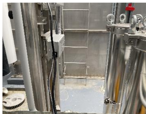
17. Interior, Level 51, Plant Room, Rain Water Tank – Rung to-ground spacing was observed to be less than 90% of the rung-to-rung spacing.
