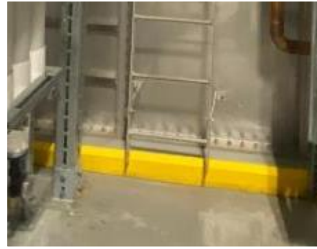
14. Interior, Level 26, Plant Room, Rain Water Tank – The concrete platform, located beneath the tank, was observed to impede the required 200 mm clearance from the back edge of the rungs of the rung ladder.
