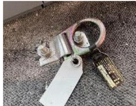
8. Level 17, Balcony – Certification tag of internal anchor point indicates annual inspection was due June 2022.
