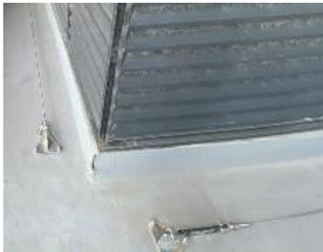
9. Exterior, Podium 3, Plant Room, Balcony – Two (2) horizontal lifeline systems were not provided with certification tags
