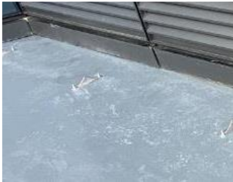
7. Exterior, Level 51, Rooftop – Several anchor points not provided with certification tags.
