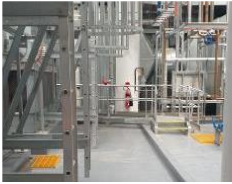
13. Interior, Level 51, Plant Room, Cooling Towers, Upper Level – Rung to-ground spacing was observed to be greater than the rung-rung spacing.
