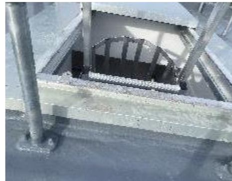
10. Exterior, Level 52, Rooftop, Upper Level - No upper landing platform provided. Uneven surface surrounding the access hatch presenting a trip hazard.
