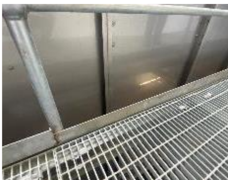
11. Interior, Level 51, Plant Room, Upper Level – Unsecured toe board presenting a risk of falling objects.
