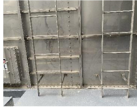
18. Interior, Level 51, Plant Room, Potable Water Tank – Rung to-ground spacing was observed to be less than 90% of the rung-to-rung spacing.
