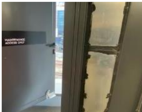
3. Exterior, Podium 3, Plant Room, Balcony – The lock provided to the door to the balcony was faulty, leaving the door unsecured.
