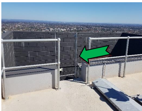
1. Upper Rooftop – The roof was provided with a rung ladder, with stiles extending approximately 1,000 mm, for access.
