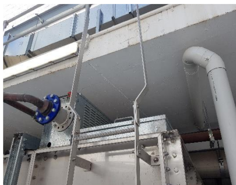
5. Level 34, Mechanical Plant Room – Restricted head height at the top of the Potable Drinking Water Tank.
