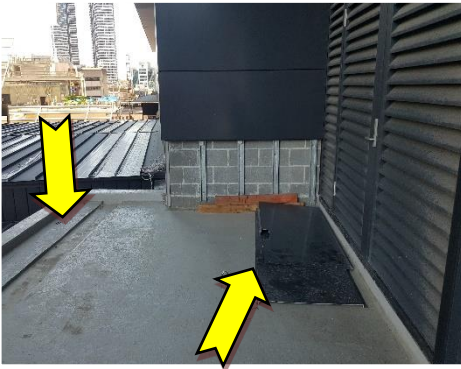
9. Podium 3, Western Elevation Roof – Glass Safe Weight Limit was not displayed and building materials were observed to obstruct the entrance.
