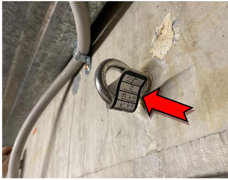
7. Level 1, OSD tank – The inspection tags for the anchor points at the top of the tank were observed to be out of date.
