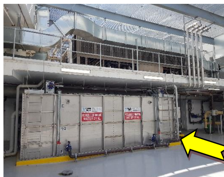
6. Level 34, Mechanical Plant Room – The pipework at the base of the western ladder was observed to obstruct the rear ladder clearance.
