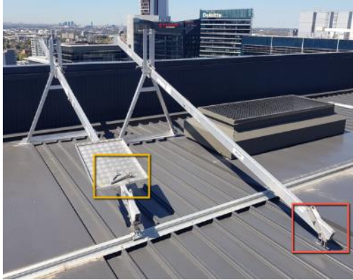
Figure 1: Rooftop, South-Eastern Corner – A needle was observed to be unsecured (red) and minor components were observed to be stored on a needle system (yellow) (left).
