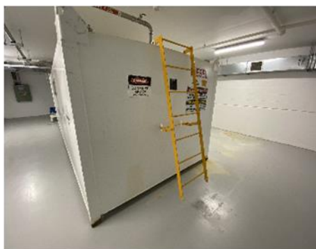
Figure 16: Level B3, Plant Room, Diesel Storage Tank – Rung ladder provided to access the dip point of the diesel storage tank.
