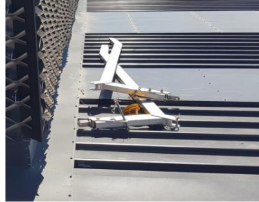
Figure 2: Loose fall arrest equipment was observed to be stored adjacent the needle systems (right).
