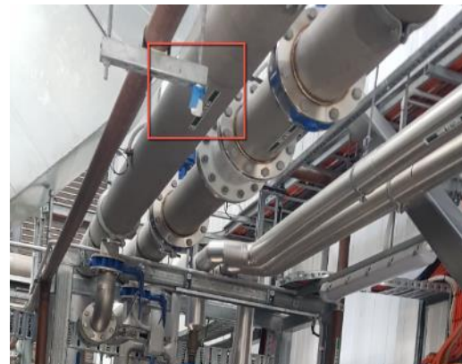
Figure 10: Level 17, Cooling Tower Plant Room – Low headroom was observed on a platform walkway adjacent to the cooling towers due to the presence of pipework and a bracket.
