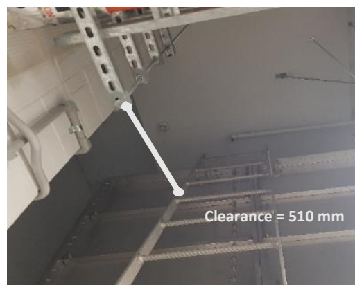
Figure 14: Level 2 Plant Room, OSD Tank – The front clearance was measured to be 510 mm due to protruding metal brackets located adjacent to the ladder.
