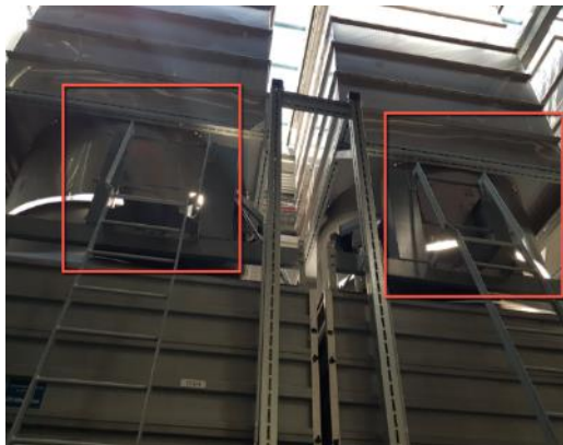
Figure 9: Level 17, Cooling Tower Plant Room – The gates provided to access cooling towers were noted to be difficult to open which may increase the risk of falls.
