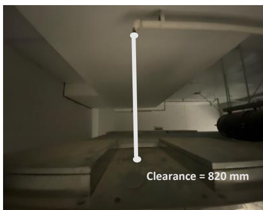
Figure 13: Level 2 Plant Room, OSD Tank – the landing headroom provided at the top of the rung ladder was measured to be 820 mm high.
