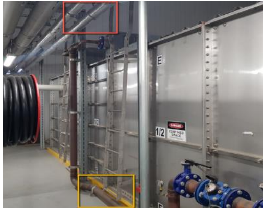
Figure 7: Level 17, Plant Room, Water Tank Area – A metal pipe beneath the bottom rung was considered to pose a trip hazard when descending the rung ladder (yellow) and head clearance was noted to be obstructed by HHW Flow and HHW return pipework (red).
