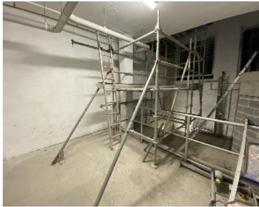
Figure 15: Level B2, Plenum, Authorised Access Only Room – Scaffolding erected to provide access to an area impacted by reoccurring issues of water ingress.
