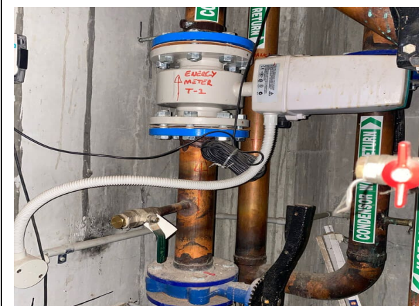
5. Pipework - Asbestos - Negative
