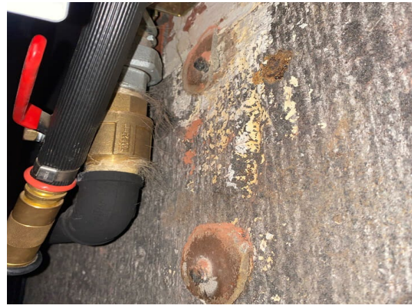
10. East side, under fire hose reel, residue on wall - Asbestos - Negative
