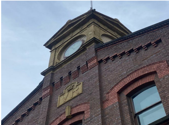
13. Clock tower - Asbestos - No Access
