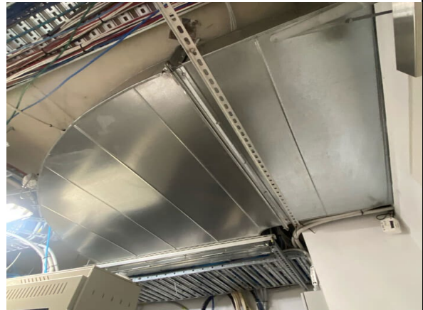
4. Ductwork, flanges - Asbestos - Negative
