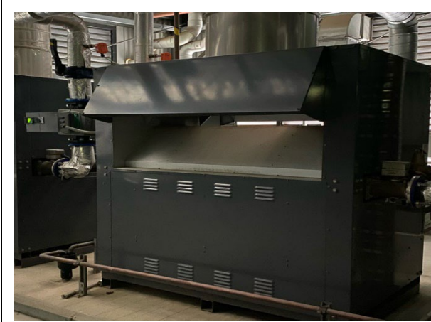
3. Australian Manufactured Boilers, internal lining - Asbestos - Negative
