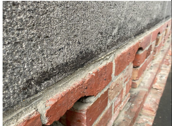
16. External west wall, bottom of stone course - Asbestos - Negative
