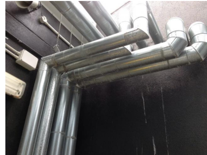
PHOTO NO.: J144435-APS-PRO-059-PHOTO002 RESULT: SMF - POSITIVE BUILDING/LEVEL: 710 COLLINS STREET (GOODS SHED NORTH) - ROOF ROOM ROOM/LOCATION: PLANT ENCLOSURE - VARIOUS THROUGHOUT FEATURE/MATERIAL: PIPEWORK INSULATION - GLASS FIBRE SAMPLE NO.: -
