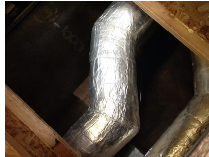
PHOTO NO.: J144435-APS-PRO-059-PHOTO018 RESULT: SMF - POSITIVE BUILDING/LEVEL: 710 COLLINS STREET (GOODS SHED NORTH) - GROUND LEVEL ROOM/LOCATION: SUBFLOOR ACCESS - WITHIN FEATURE/MATERIAL: DUCTWORK INSULATION - SARKING INSULATION SAMPLE NO.: -
