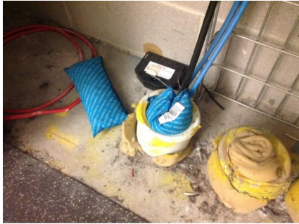
PHOTO NO.: J144435-APS-PRO-059-PHOTO010 RESULT: SMF - POSITIVE BUILDING/LEVEL: 710 COLLINS STREET (GOODS SHED NORTH) - ALL LEVELS ROOM/LOCATION: ELECTRICAL RISERS - GENERAL THROUGHOUT FEATURE/MATERIAL: PENETRATIONS - PILLOW INSULATION SAMPLE NO.: -
