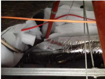
PHOTO NO.: J144435-APS-PRO-059-PHOTO013 RESULT: SMF - POSITIVE BUILDING/LEVEL: 710 COLLINS STREET (GOODS SHED NORTH) - LEVEL TWO ROOM/LOCATION: CEILING SPACE - OFFICE AREAS FEATURE/MATERIAL: FLEXIBLE DUCTWORK INSULATION - SARKING INSULATION SAMPLE NO.: -
