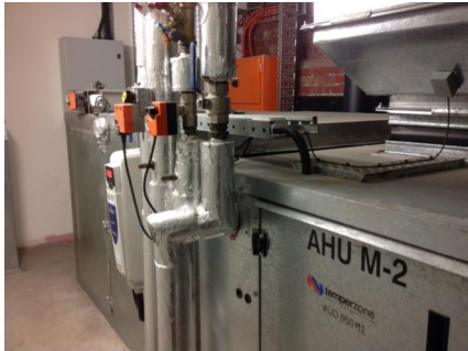
PHOTO NO.: J144435-APS-PRO-059-PHOTO017 RESULT: SMF - POSITIVE BUILDING/LEVEL: 710 COLLINS STREET (GOODS SHED NORTH) - GROUND LEVEL ROOM/LOCATION: AIR HANDLING PLANT ROOMS X 6 - THROUGHOUT FEATURE/MATERIAL: PIPEWORK INSULATION - SARKING INSULATION SAMPLE NO.: -
