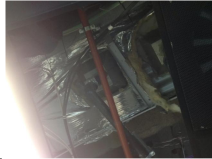
PHOTO NO.: J144435-APS-PRO-059-PHOTO009 RESULT: SMF - POSITIVE BUILDING/LEVEL: 710 COLLINS STREET (GOODS SHED NORTH) - LEVEL TWO ROOM/LOCATION: CEILING SPACE - OFFICE AREAS FEATURE/MATERIAL: DUCTWORK INSULATION - SARKING INSULATION SAMPLE NO.: -
