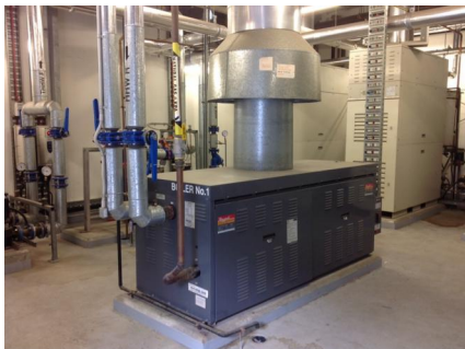
PHOTO NO.: J144435-APS-PRO-059-PHOTO005 RESULT: SMF - PRESUMED POSITIVE BUILDING/LEVEL: 710 COLLINS STREET (GOODS SHED NORTH) - ROOF ROOM ROOM/LOCATION: BOILER PLANT ROOM - CENTRAL FEATURE/MATERIAL: BOILER INSULATION - GLASS FIBRE SAMPLE NO.: -
