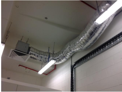
PHOTO NO.: J144435-APS-PRO-059-PHOTO014 RESULT: SMF - POSITIVE BUILDING/LEVEL: 710 COLLINS STREET (GOODS SHED NORTH) - MEZZANINE LEVEL ROOM/LOCATION: SECURITY OFFICE - CEILING AREAS FEATURE/MATERIAL: FLEXIBLE DUCTWORK INSULATION - SARKING INSULATION SAMPLE NO.: -
