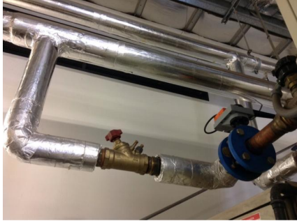
PHOTO NO.: J144435-APS-PRO-059-PHOTO011 RESULT: SMF - POSITIVE BUILDING/LEVEL: 710 COLLINS STREET (GOODS SHED NORTH) - ROOF ROOM/LOCATION: BOILER PLANT ROOM - VARIOUS THROUGHOUT FEATURE/MATERIAL: PIPEWORK INSULATION - SARKING INSULATION SAMPLE NO.: -
