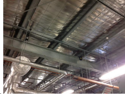
PHOTO NO.: J144435-APS-PRO-059-PHOTO004 RESULT: SMF - POSITIVE BUILDING/LEVEL: 710 COLLINS STREET (GOODS SHED NORTH) - ROOF ROOM/LOCATION: CHILLER PLANT ROOM - THROUGHOUT FEATURE/MATERIAL: CEILING - SARKING INSULATION SAMPLE NO.: -
