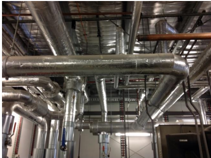
PHOTO NO.: J144435-APS-PRO-059-PHOTO012 RESULT: SMF - POSITIVE BUILDING/LEVEL: 710 COLLINS STREET (GOODS SHED NORTH) - ROOF ROOM/LOCATION: CHILLER PLANT ROOM - VARIOUS THROUGHOUT FEATURE/MATERIAL: PIPEWORK INSULATION - GLASS FIBRE SAMPLE NO.: -
