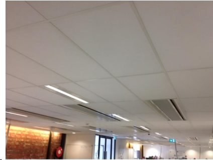
PHOTO NO.: J144435-APS-PRO-059-PHOTO008 RESULT: SMF - POSITIVE BUILDING/LEVEL: 710 COLLINS STREET (GOODS SHED NORTH) - ALL LEVELS ROOM/LOCATION: OFFICE AREAS - VARIOUS THROUGHOUT FEATURE/MATERIAL: CEILING TILES - COMPRESSED CEILING TILES SAMPLE NO.: -
